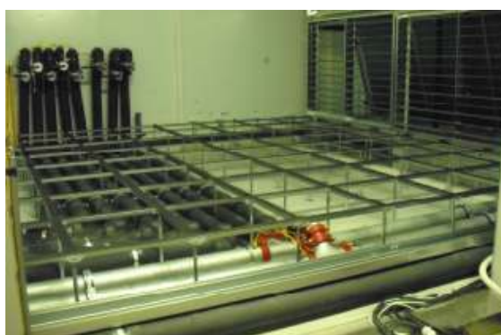
Hydraulic pipeworks in raised floor
